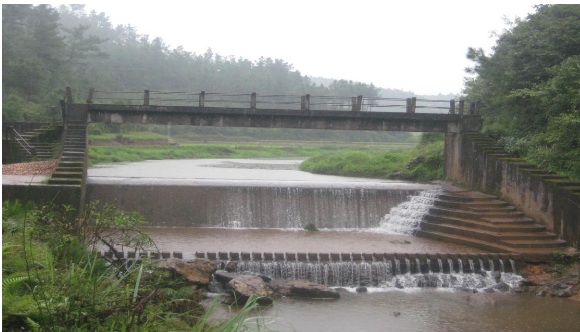
Views of Headwork from the downstream at Krang Umsier Flow Irrigation Project
